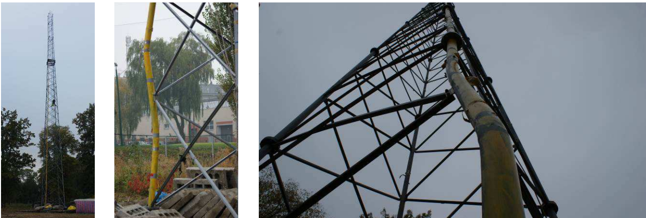
Figure 1. The general view of the tower (left), failure mode of the leg in the lowest section (middle and right)
